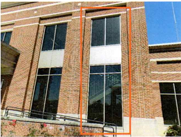
5. Window leak location 1 (WL1). East of entrance to the Administrative Building.
