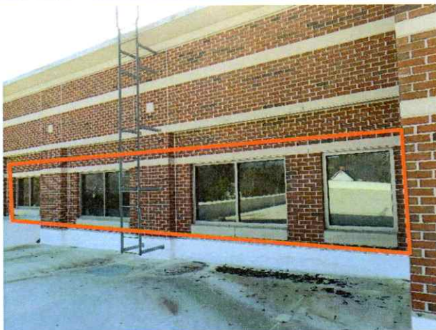
15. Reported leaks at roof level windows on the north elevation of the Courts Building (WL3).
