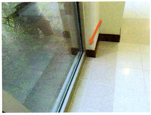
14. Water staining at adjacent wall base to WL2.
