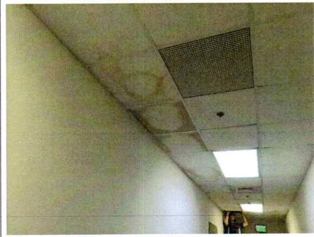
18. Water staining at interior corridor ceiling tiles related to TL1.
