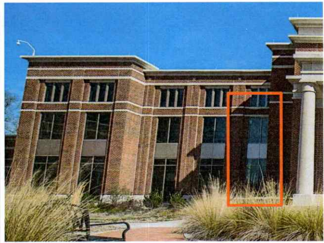
10. Window leak location 2 (WL2). North of entrance to the Courts Building.
