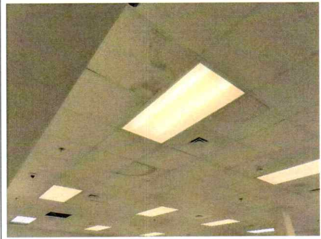
34. Series of plumbing leaks (PL3) within the Records Room on the first floor.
