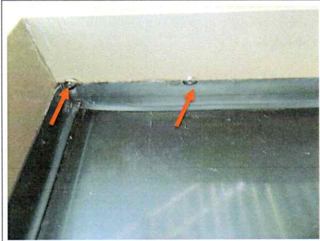
7. Water leak testing revealed water intrusion through window seals at WL1.
