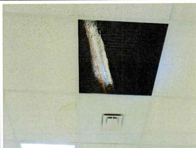
35. Series of plumbing leaks (PL3) within the Records Room on the first floor.
