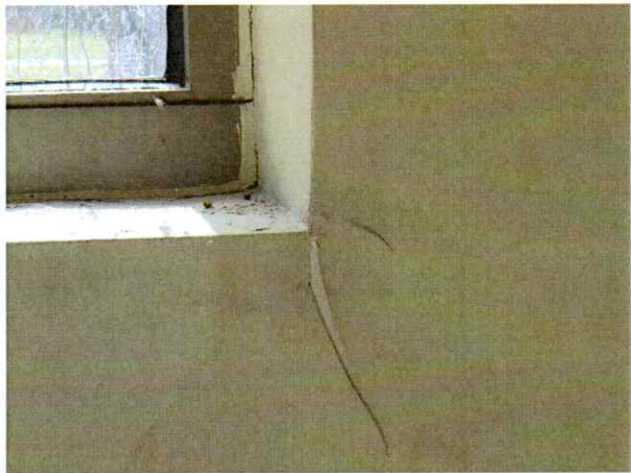
9. Water staining and peeling paint from long-term water intrusion at WL1 interior wall.
