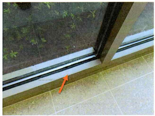
12. Water leak testing revealed pooling water at the base of the center mullion at WL2.
