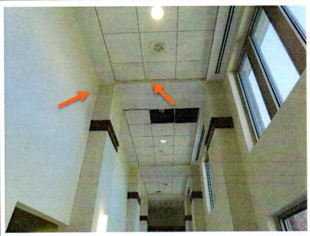
32. Series of plumbing leaks (PL2) on the second floor outside the District Attorney's office.
