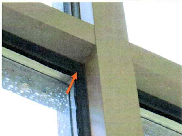
11. Water leak testing revealed water intrusion through center mullion at WL2.
