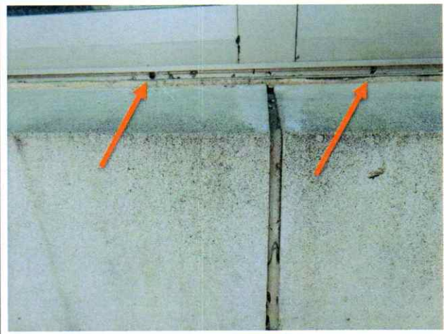
16. Typical condition of WL3 windows. Retrofitted weep holes in windowsills.
