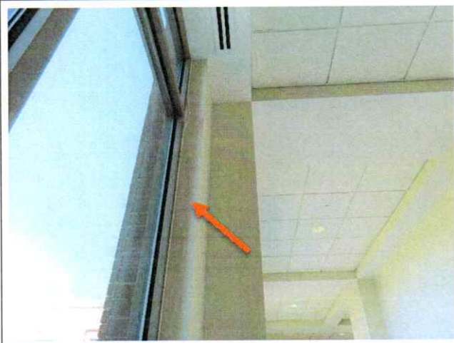
13. Water staining at adjacent wall to WL2.
