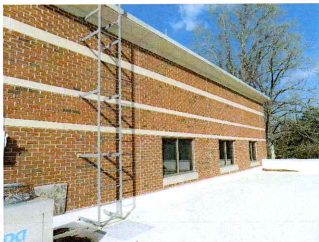
17. Wall above roof transition leak 1 (TL1).
