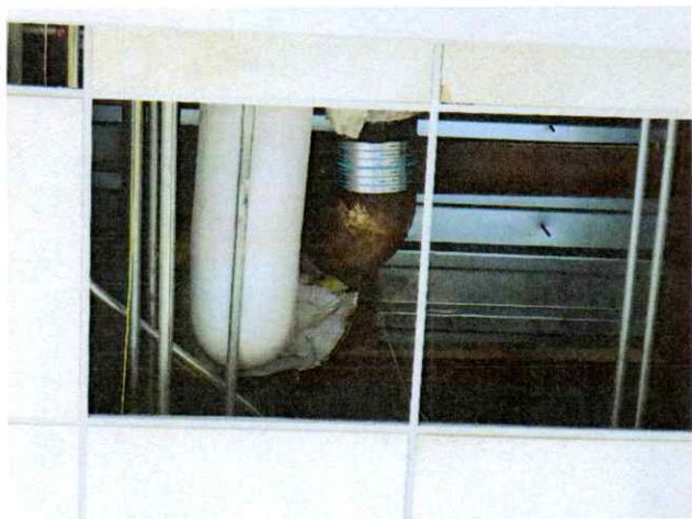
33. Severely corroded drainage pipe with replaced 3-band no-hub coupling related to PL2.
