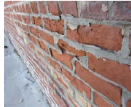
Historic masonry that has been repointed with Portland cement which has led to degradation.
